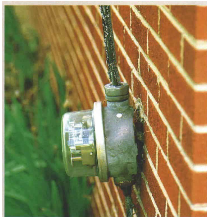
Clues to what lies beneath. Besides its dubious attachment to the wall, small meter bases such as this one are made to handle 60 amps and should not be supplying a 150-amp or 200-amp service panel.
