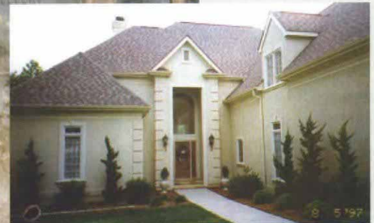
Be wary with stucco finishes. It pays to be careful when inspecting a house with a stucco exterior. From the outside, nothing seems wrong with this barrier-type synthetic-stucco exterior (inset). Inside the wall, it's a different story.
