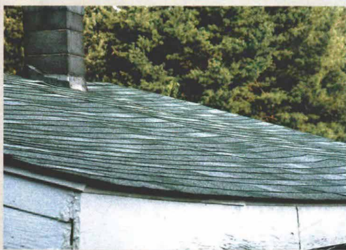
A roof should be straight. A wavy roof deck can indicate that the underlying sheathing is too thin or starting to rot or delaminate. A sagging ridge may mean the same thing.
